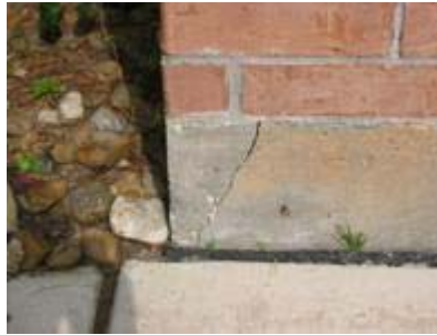
corner or wedge crack
