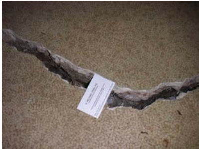
this is a very wide crack that has faulted severely; notice the business card
