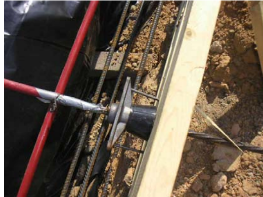
close-up showing a live-end anchor; notice the use of duct tape – this shows poor workmanship
